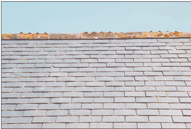
Above: Careful re-use of its ridge tiles has meant this roof has retained most of its historic interest and character even though the slates themselves required renewal. The appearance and hand-made qualities of the tiles are a positive asset.
